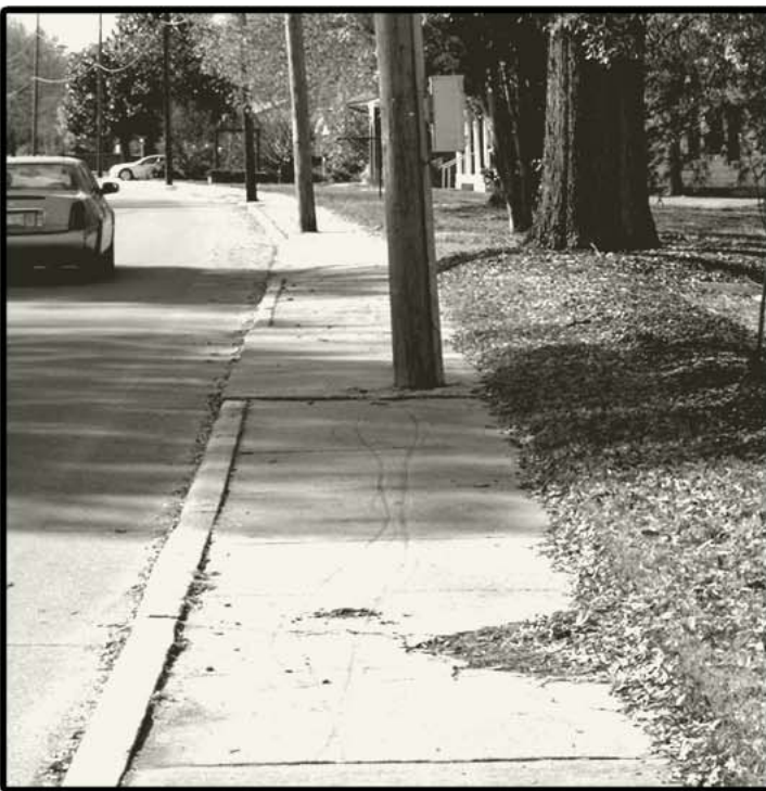
Many Cherryville sidewalks present obstacles, particularly to the physically challenged, as they are blocked by obstructions and are in need of repair.
